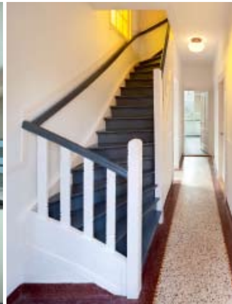
Wooden stairs and terrazzo floors have been preserved in their original condition.
